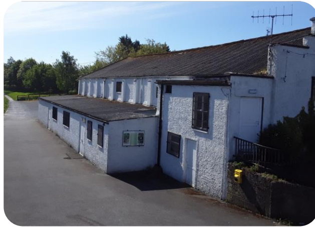
A noticeable sag in the roof bespeaks structural damage...
